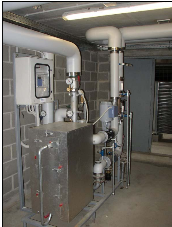
View of a building substation.
